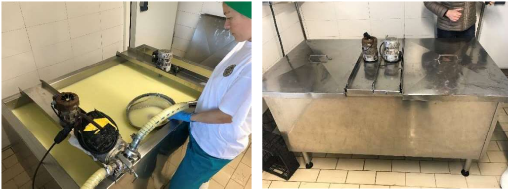
Figure 5.10: Raw milk coagulation process: Heated tank with the two mixers on its top for cutting
